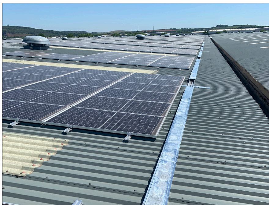
Figure 5.7.1 Module installation nearing completion (Reproduced by kind permission of Chris Roberts, Clean Energy Consulting Ltd)
