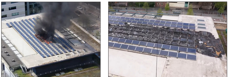
Figure A6.6 Solar panel fire on roof of Bristol science museum, April 2022. Due to damage, the museum will not reopen until 2023 (Source: Avon & Somerset Constabulary drone footage)
